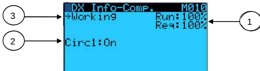
Figure_7.3 Main monitoring page 3 - Compressor statuses
