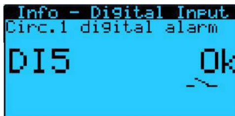
Figure 7.10: Digital input terminal DI5 - Digital alarm for the 1st Circuit
